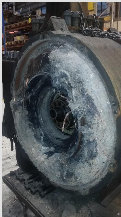
Figur 8: Demontert endedeksel. Skadet vikling. Foto: CargoNet AS
